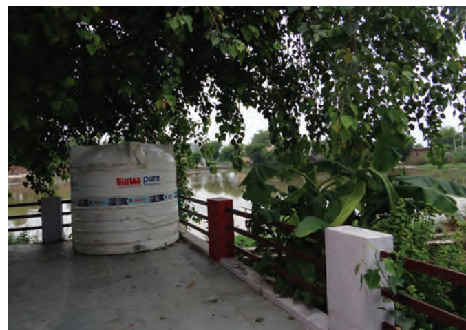
Water Tank @Site Picture
