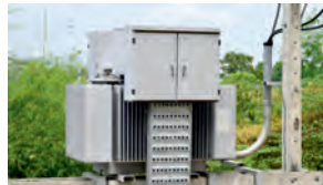
LOW TENSION ELECTRIC WORK
