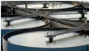
SEWAGE TREATMENT PLANTS
