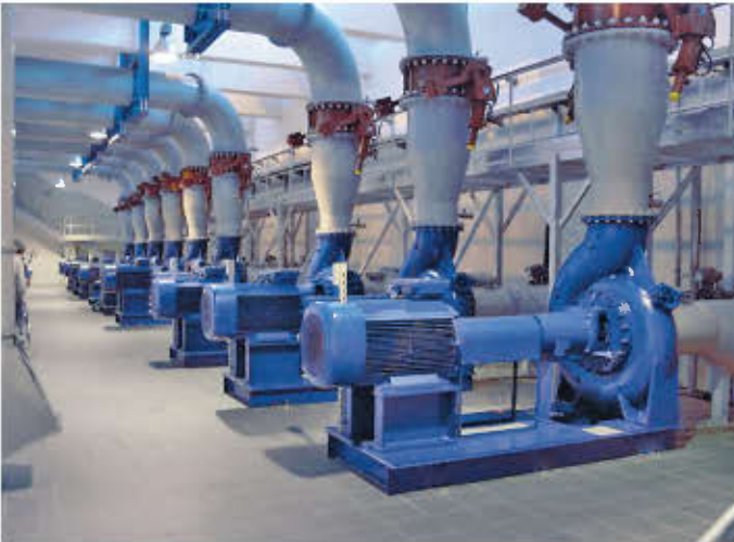
Water Pumping System
