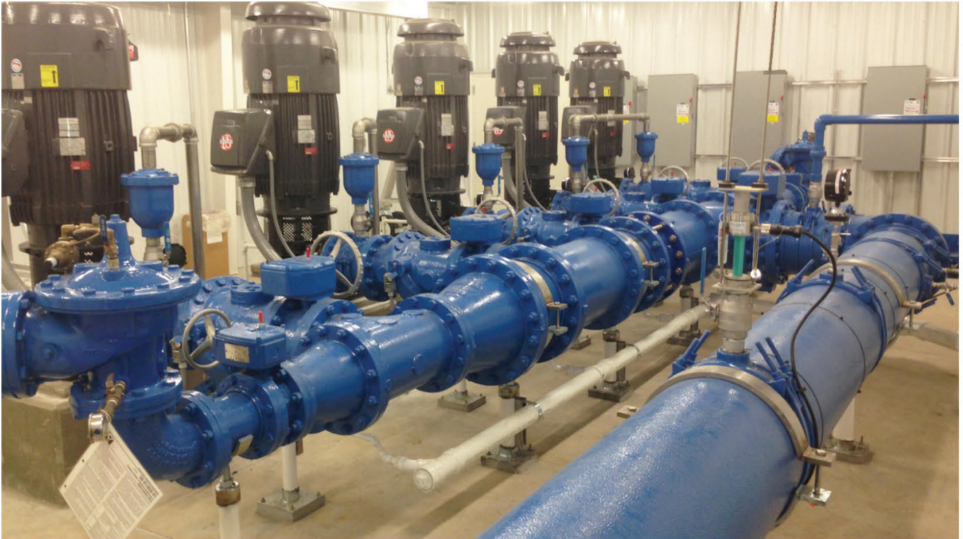
Pumping Station for Drinking Water Supply
