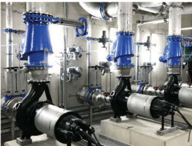
Water Supply Pumping System
