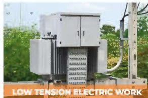
LOW TENSION ELECTRIC WORK
