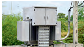
LOW TENSION ELECTRIC WORK
