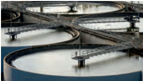
SEWAGE TREATMENT PLANTS
