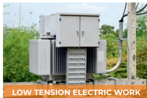
LOW TENSION ELECTRIC WORK
