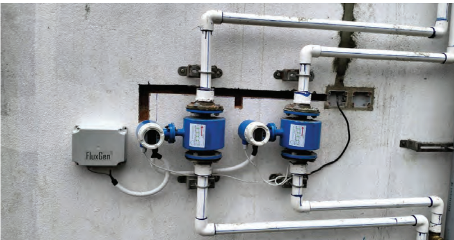
Smart water meters connected to pipelines.
