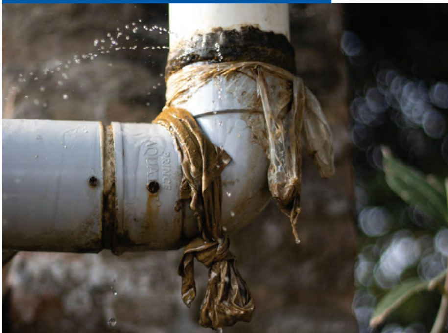
Leakages and pipe breakages substantially increase the cost of water to industries.
