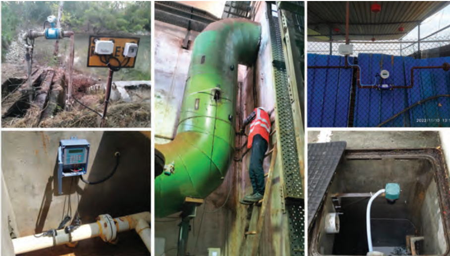
Installations of water meters and other equipment in the facility.
