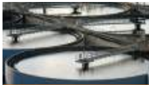
SEWAGE TREATMENT PLANTS
