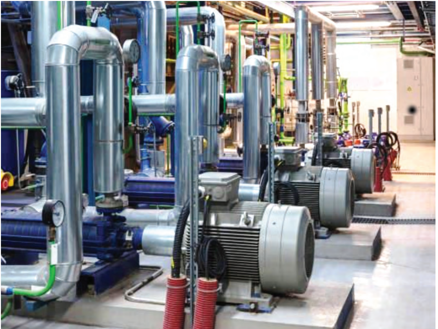
Industrial Liquid Supply Pumping System
