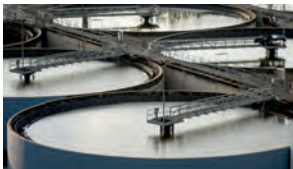
SEWAGE TREATMENT PLANTS
