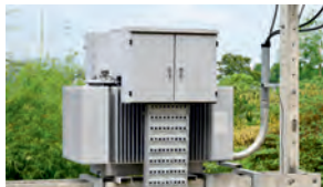
LOW TENSION ELECTRIC WORK
