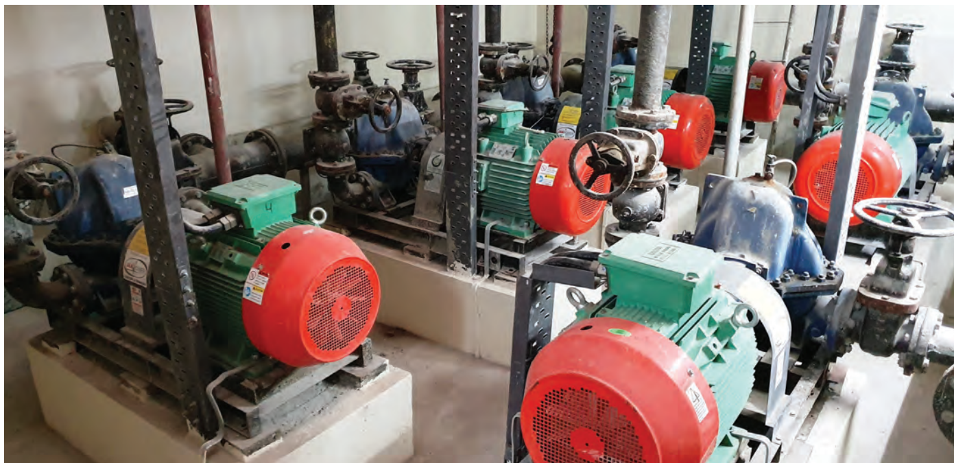
Booster Pumping Station, Narela, Delhi
