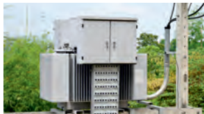
LOW TENSION ELECTRIC WORK
