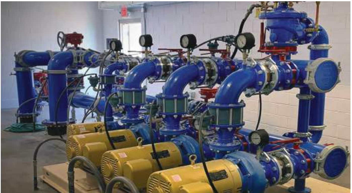
Water Pumping Station
