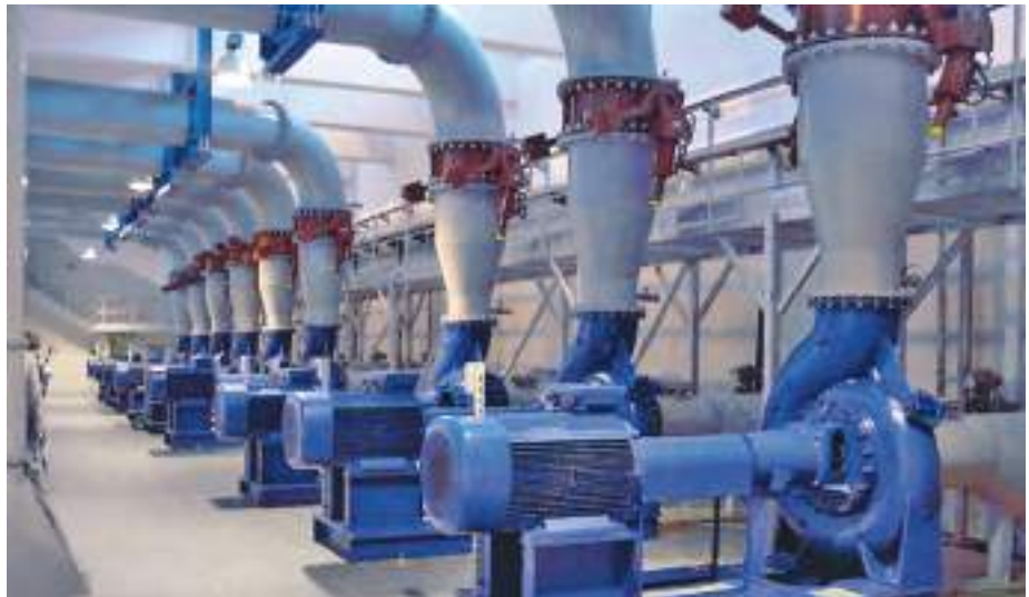
Water Pumping System
