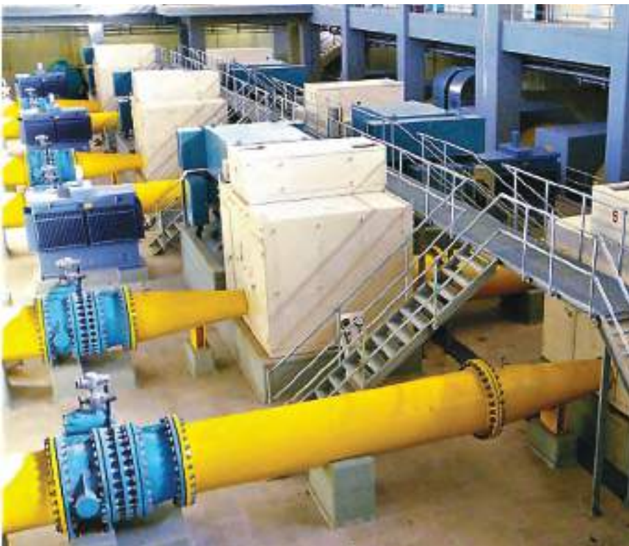
Water Pumping System for Drinking Water Supply
