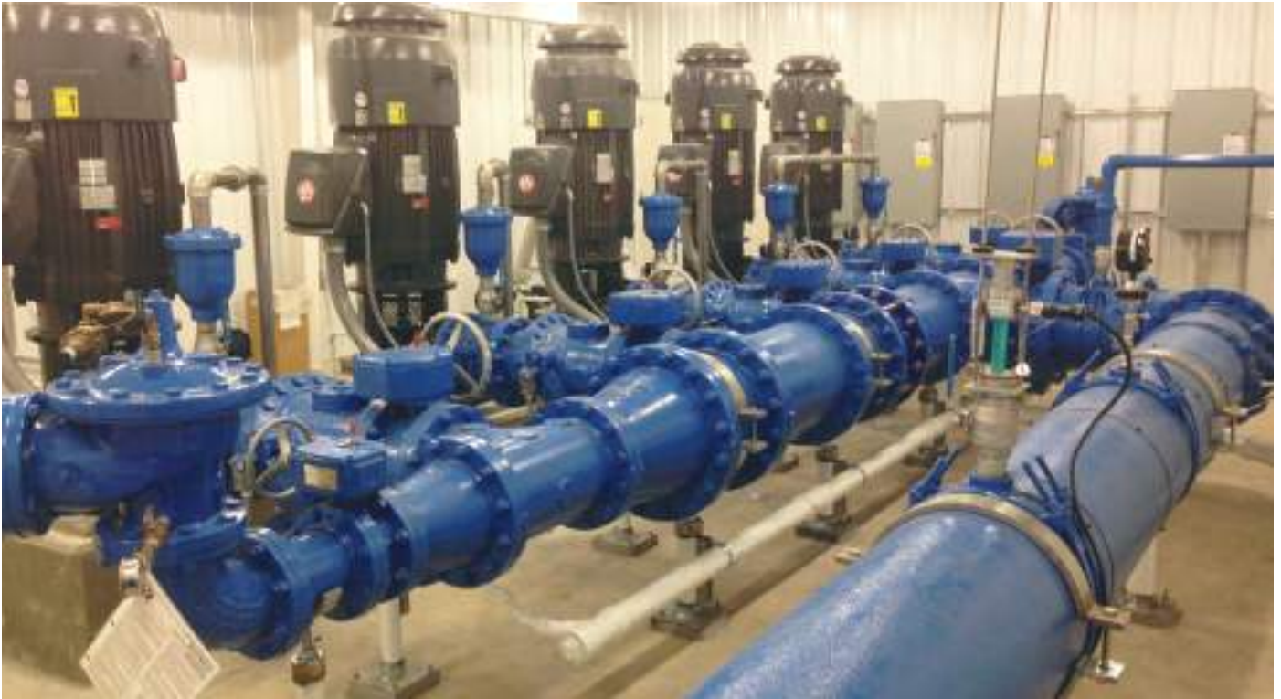
Water Pumping Station
