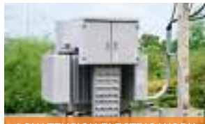
LOW TENSION ELECTRIC WORK
