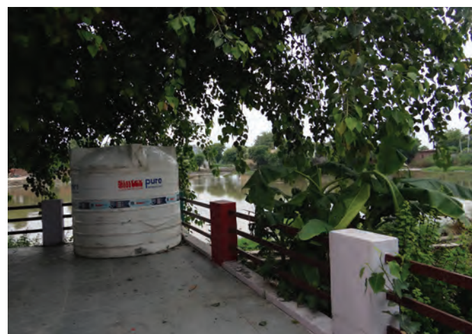
Water Tank @Site Picture
